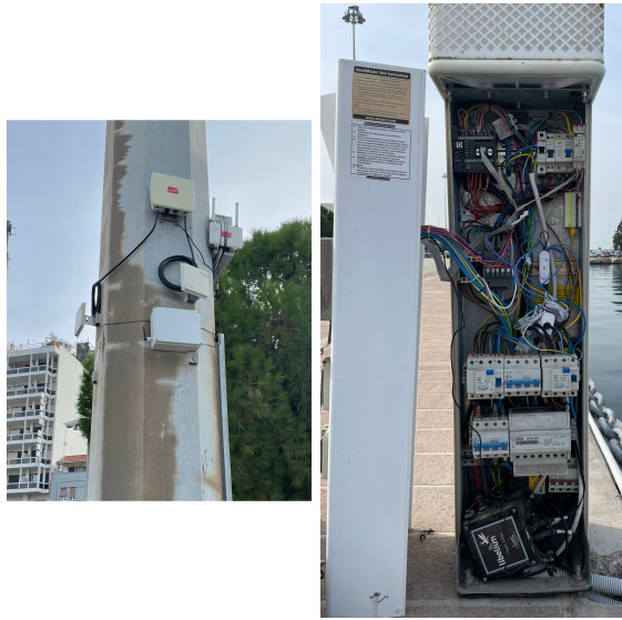
Fig. 6. Sparks Edge device installed on-site and modernized Mooring Pillar with Sparks 433-Bridge device and Shelly 3EM
